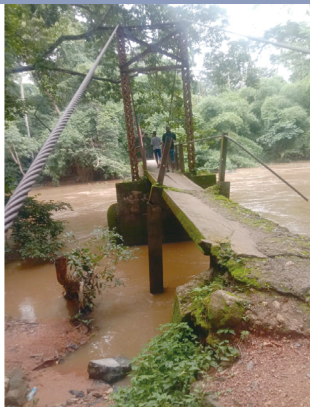
Collapsed section of the metal handrail of the suspended bridge.
